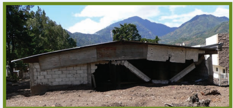
Figure 2: Effect of landslide from tropical storm Stan.
